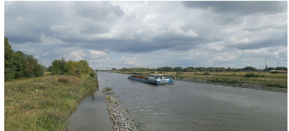
Landscaping of the riverbanks along Section 140 of the river Lys (Crédits : @DVW)
