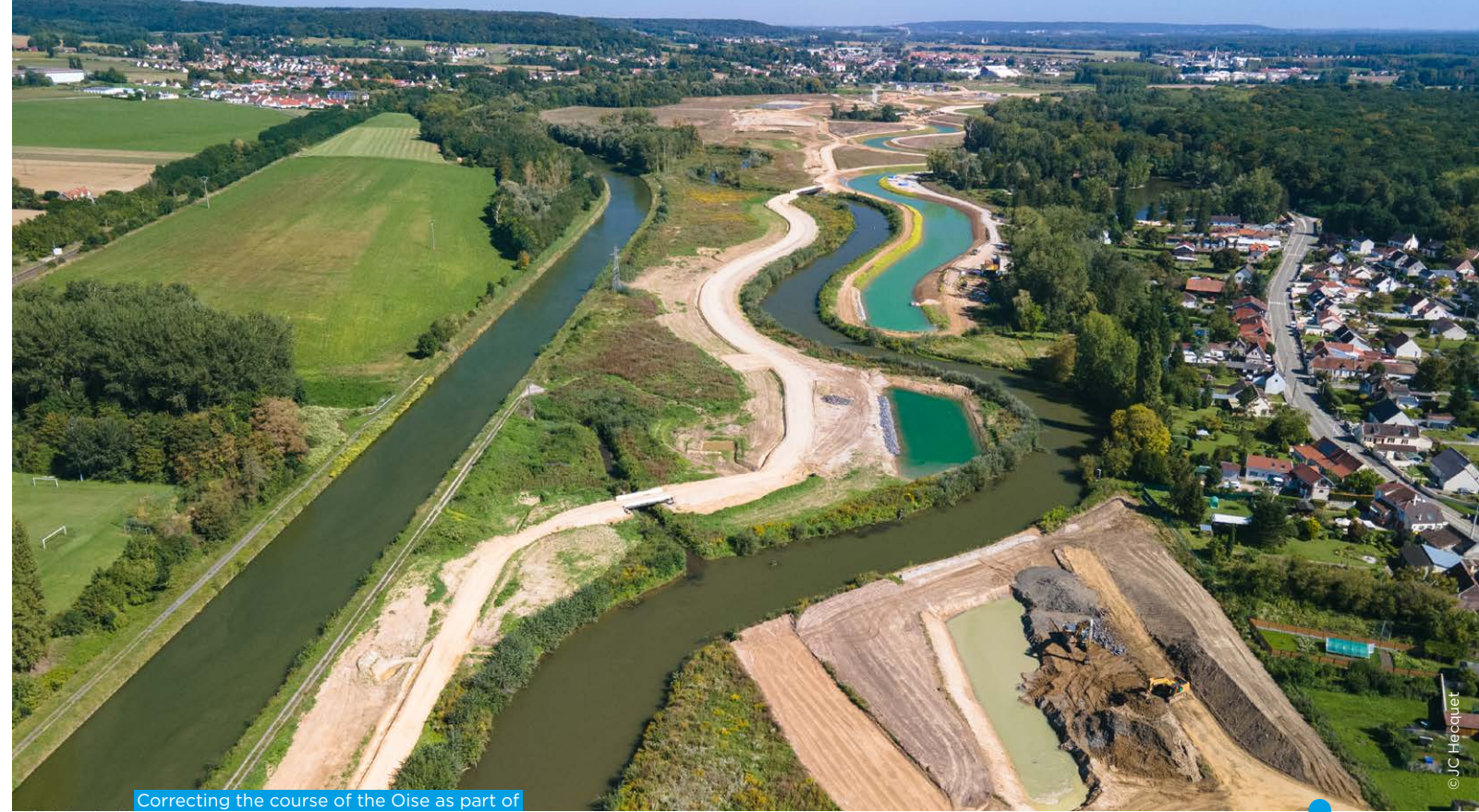
Correcting the course of the Oise as part of the construction of the Seine-Nord Europe Canal
