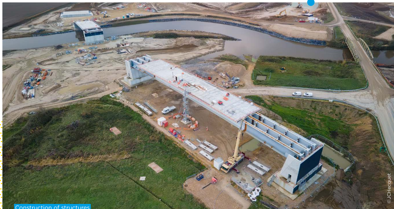
Construction of structures as part of correcting the course of the Oise
